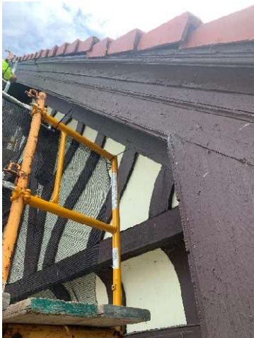
South face looking up just prior to section of roof edge being removed by Hale Roofing – 6/20/23
