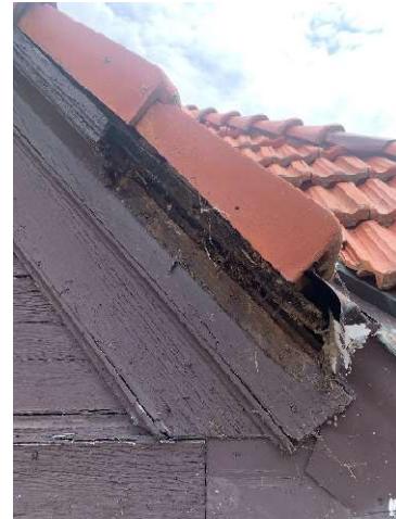
Section of existing roof edge removed by Hale Roofing to use as template – 6/20/23
