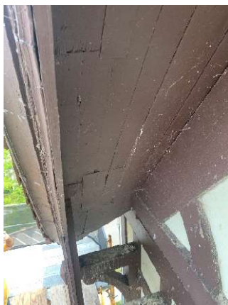
Soffit condition at North Side looking down and north. Roof edge & fascia on left of picture – 6/20/23
