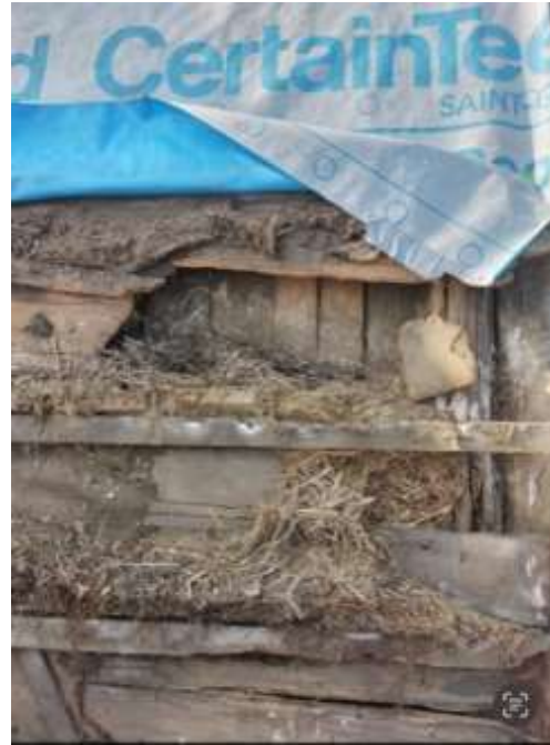
Sub-Roof Condition over soffit at North Face of West Gable
