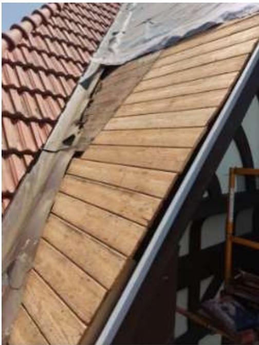
New tongue & groove cedar subroof over soffit at North Face of West Gable
